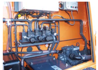
All control units tucked away in machine house under the motto "well protected, but easily accessible".
